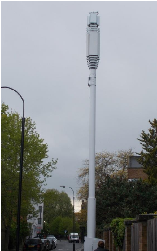
Pic: A similar mast in the borough; bulky cabinets not shown.
